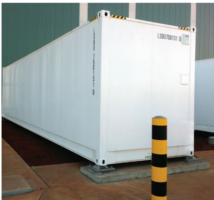
Pictured as workshop bulk lubricant storage tank
