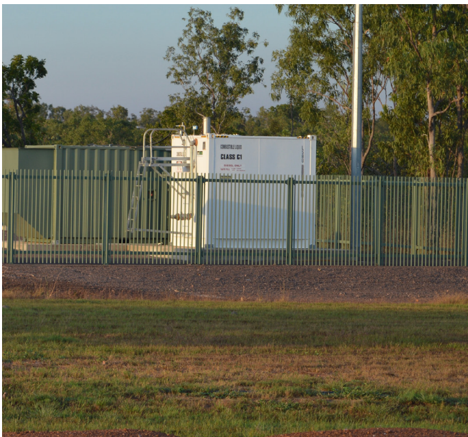
Pictured refuelling a pumping station
